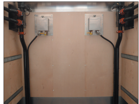
Inbox tote piping manifold system.
