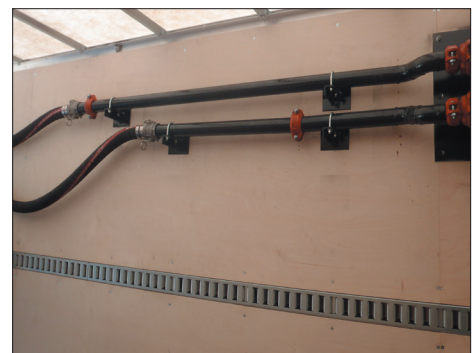
Side piping option to reach totes on the other end of the box.
