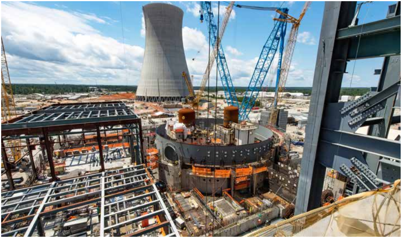
Source: Georgia Power Company via Bechtel
