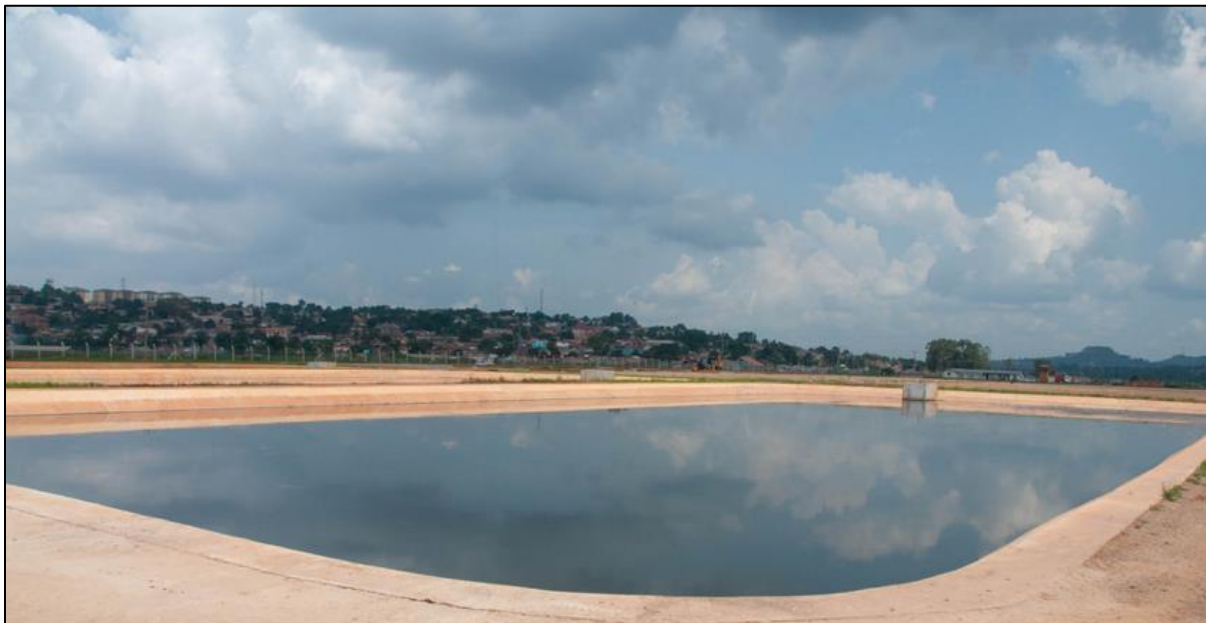
Waste stabilization ponds are a common effluent treatment technology for faecal sludge, here from settling-thickening tanks and drying beds in Kampala, Uganda. (Credit: Eawag-Sandec)
