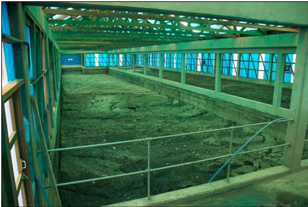
Two settling-thickening tanks in Kampala, Uganda (Credit: Lars Schoebitz)
