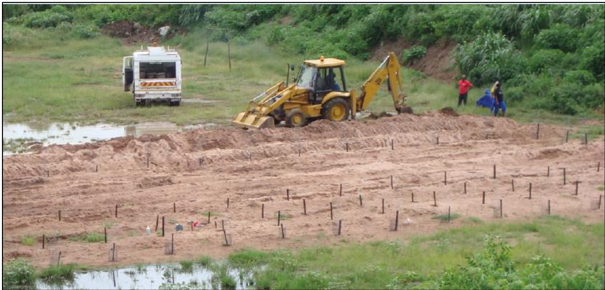
Deep row entrenchment of pit latrine faecal sludge in Durban, South Africa (Credit: Jay Bhagwan, Water Research Council South Africa in Strande et al., 2014)
