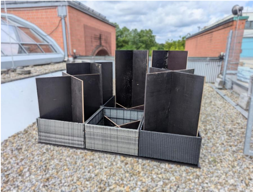
Figure 3. The Optimized Plant Building Block under construction, showing the platforms on top of which the platform, drainage layer, and soil are later placed.
